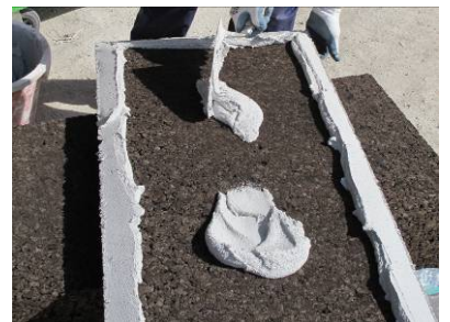
2. Applying ADHERE Vit ecoCORK on the back of the panels using the fixing method
